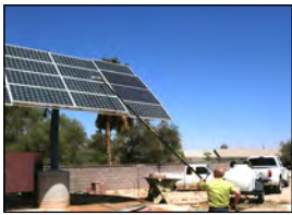
SOLAR PANEL CLEANING
