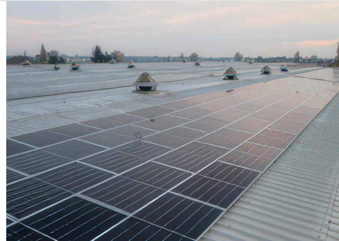
Solar panels on Italy manufacturing plant
